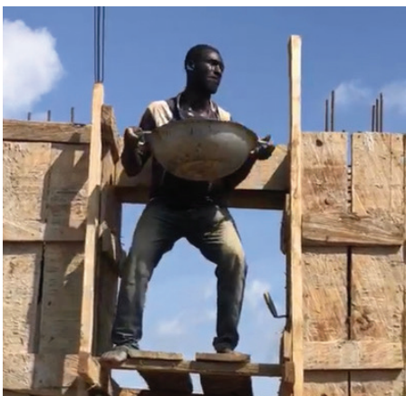
Construction workers building the wall around the ministry and vocational school land
